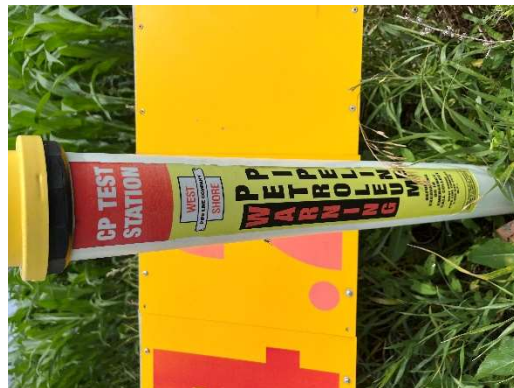
View of Petroleum Pipeline Identifier
